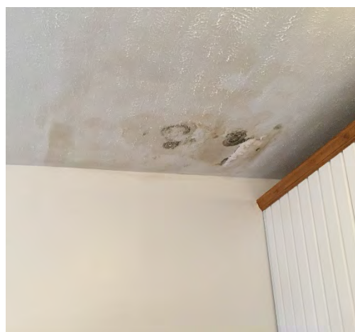
Photograph 4: Water damage and mold.
