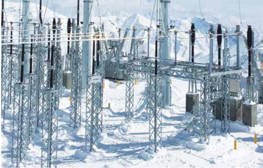
Power transformers and other infrastructure at the PTEC Salang substation. (SIGAR photo)
