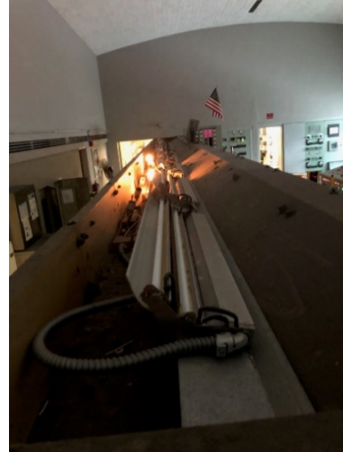
Illustration 2: Electric Control Building Control Room Emergency Lights
