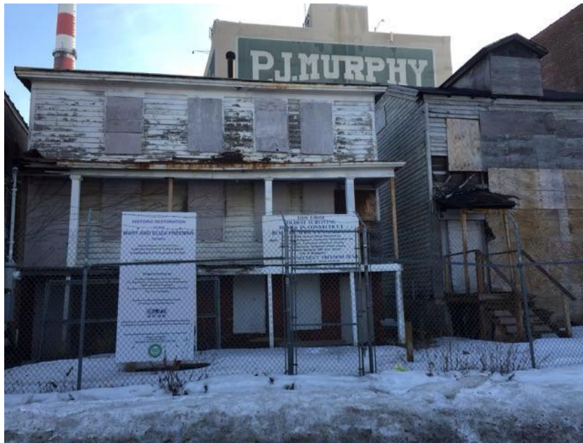
NSP funds used to stabilize property at 354 and 360 Main Street, Bridgeport, CT
