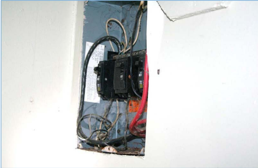
The picture above shows a missing breaker panel cover with exposed wiring, creating an electrical hazard.
