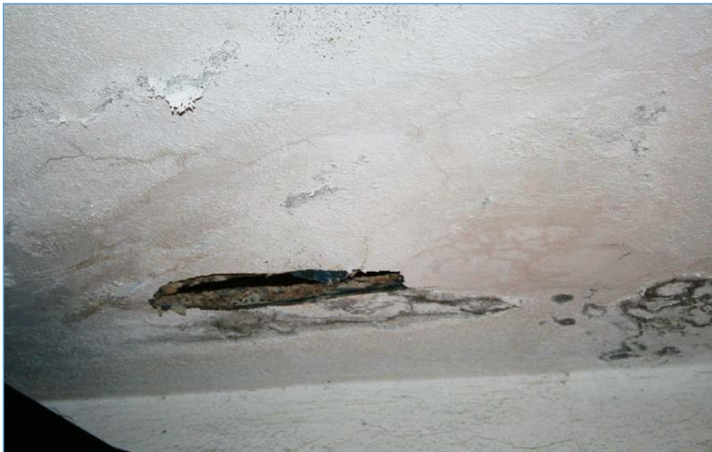
The picture above shows a water-damaged ceiling with loose plaster.
