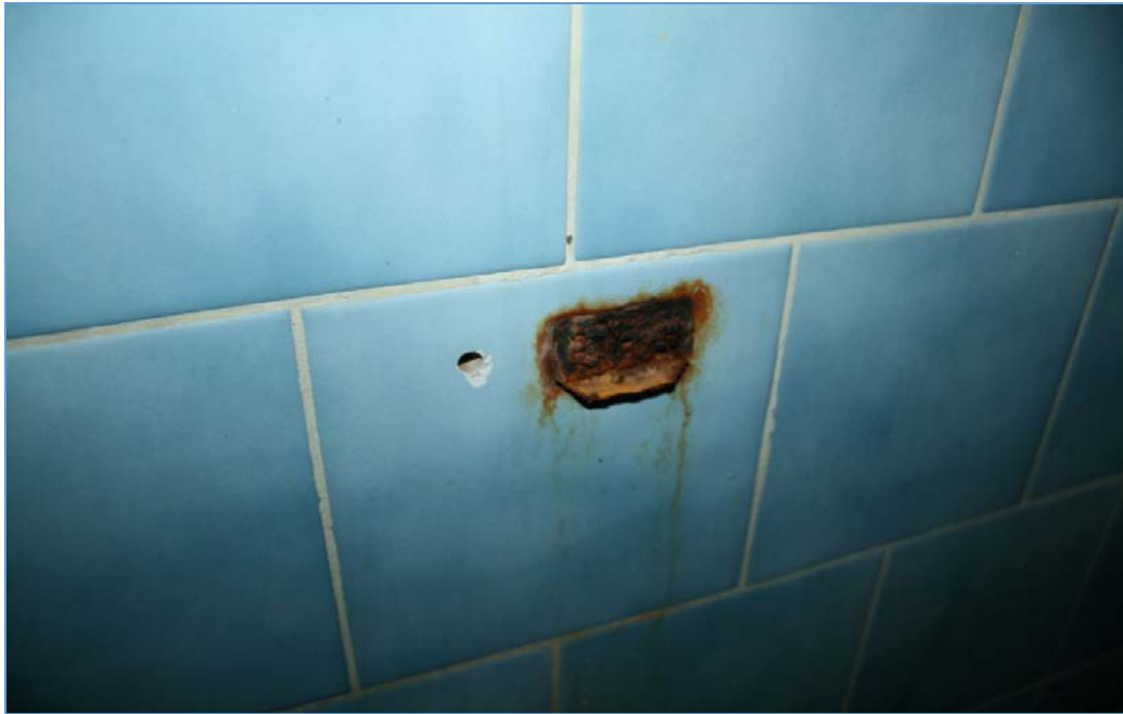
The picture above shows a missing soap dish in the shower. The rusted and sharp corners create a cutting hazard.
