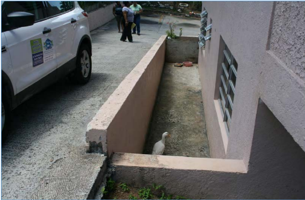
The picture above shows a retaining wall that does not have railings, creating a falling hazard. The fall distance ranges from 31 to 79 inches. A fall distance of 30 inches or more requires a railing.
