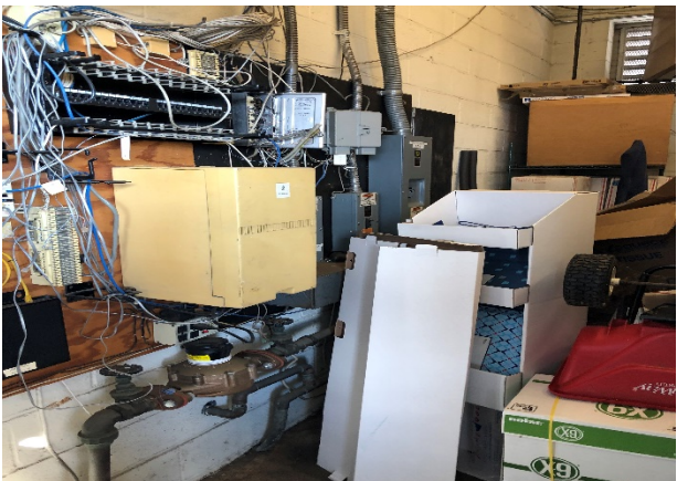
Figure 17. Blocked Electrical Panels
