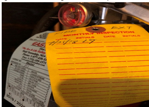
Figure 15. Fire Extinguisher not Inspected Monthly
