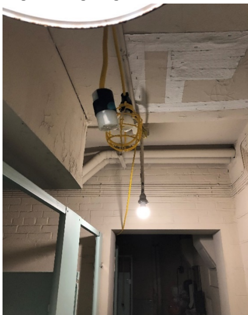
Figure 1. Lighting in Men's Restroom
