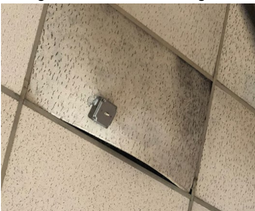
Figure 14. Unsecured Ceiling Tile
