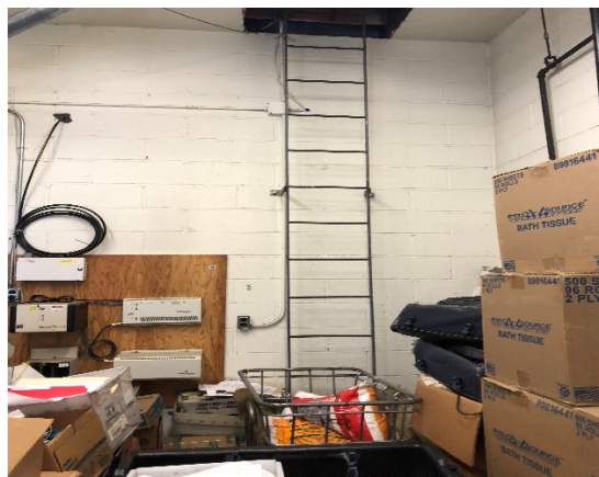
Figure 18. Blocked Ladder to Roof
