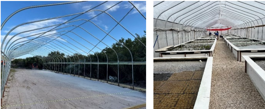
Left to right: Construction of a greenhouse at Sea and Shoreline. The completed greenhouse. (EPA OIG images)
