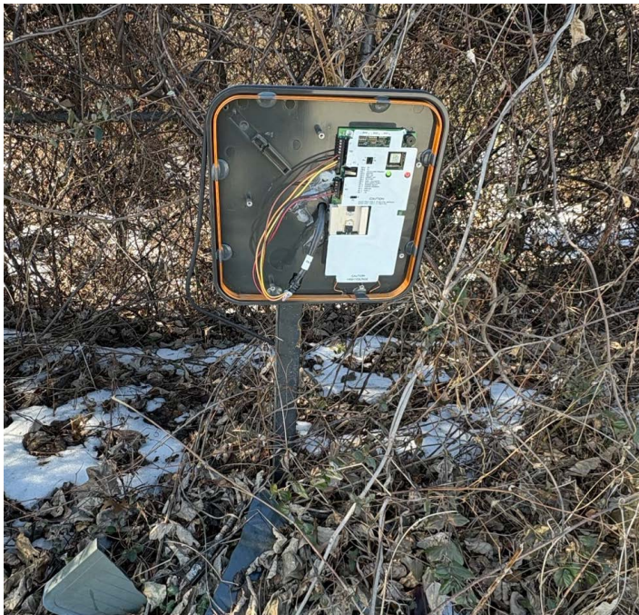
Figure 8. Broken Security Gate Control Panels at the Lynchburg MPO
