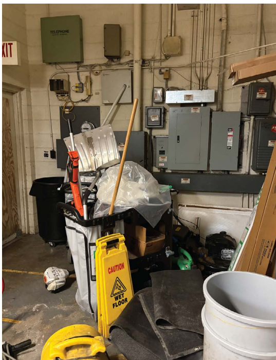
Blocked Electrical Panel
