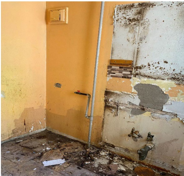
Figure 9. Peeling paint, damaged kitchen floor, mildew or mold
