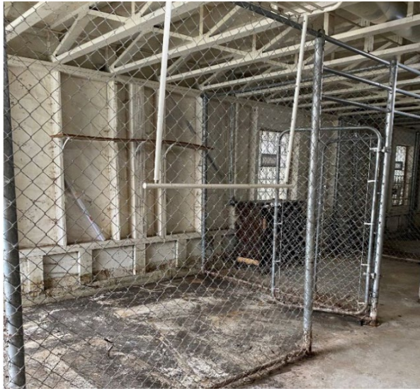
Figure 7. Unit was gutted and uninhabitable
