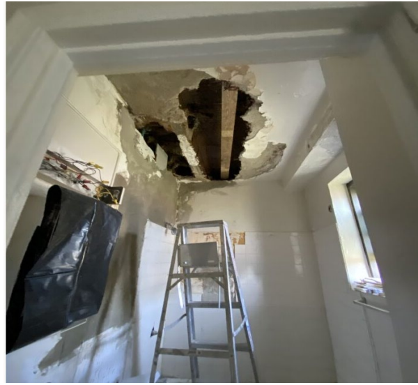
Figure 8. Unit had ceiling damage
