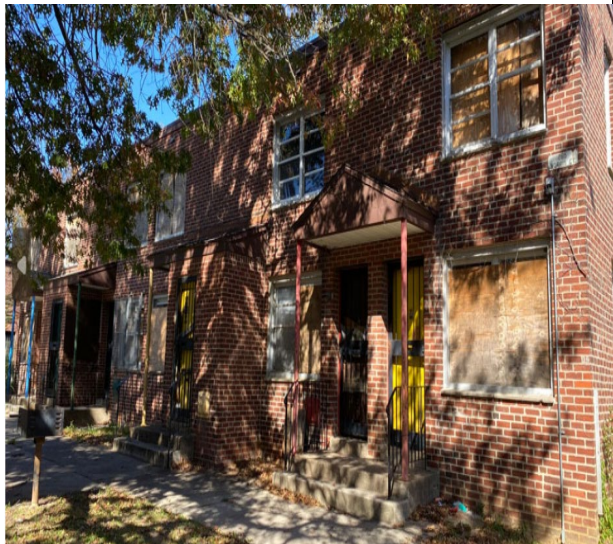
Figure 6. The entire block of eight units was vacant and uninhabitable
