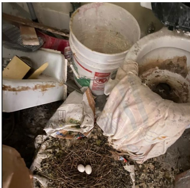
Figure 3. Bathroom damaged, bird feces and bird eggs (air quality and potential infestation)
