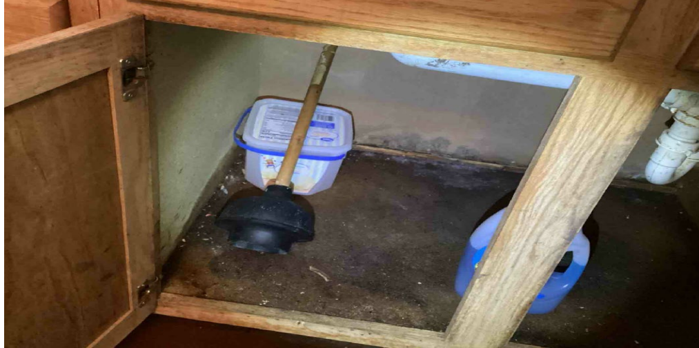
Figure 6: Photograph from RHS’ records of an inspection performed at a sample project. The photograph shows mold growth underneath a unit’s leaking kitchen sink. As of December 31, 2025, this issue has remained unresolved for 321 days after RHS notified the borrower.
