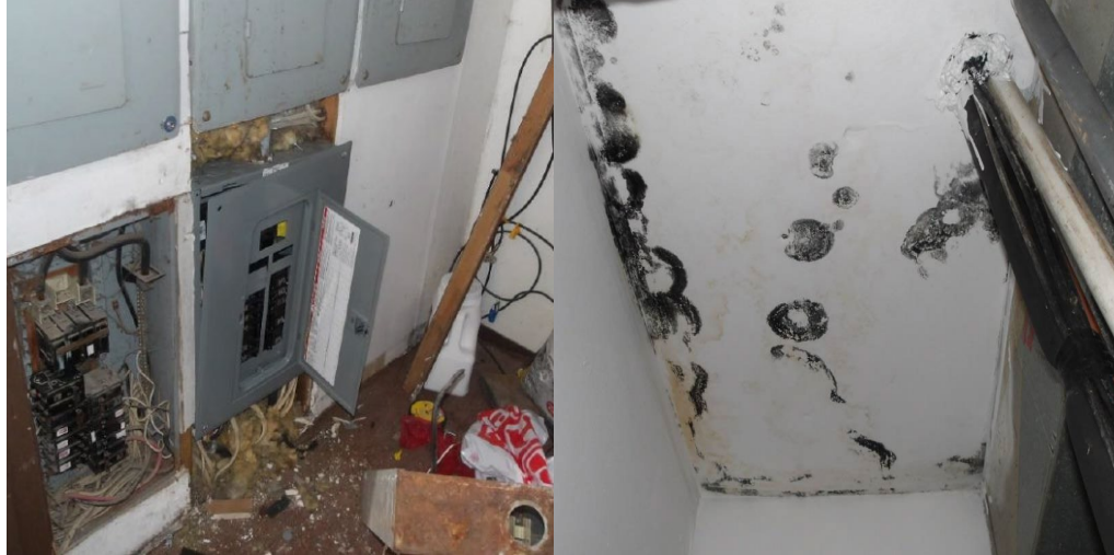
Figures 3 and 4: Photographs from RHS' records of an inspection performed at a sample project. The first photograph (left) is of a building's mechanical room showing an electrical panel with a missing cover and exposed wires. The second photograph (right) shows mold growth on a unit's ceiling. As of December 31, 2025, both issues remained unresolved for 512 days after RHS notified the borrower.
