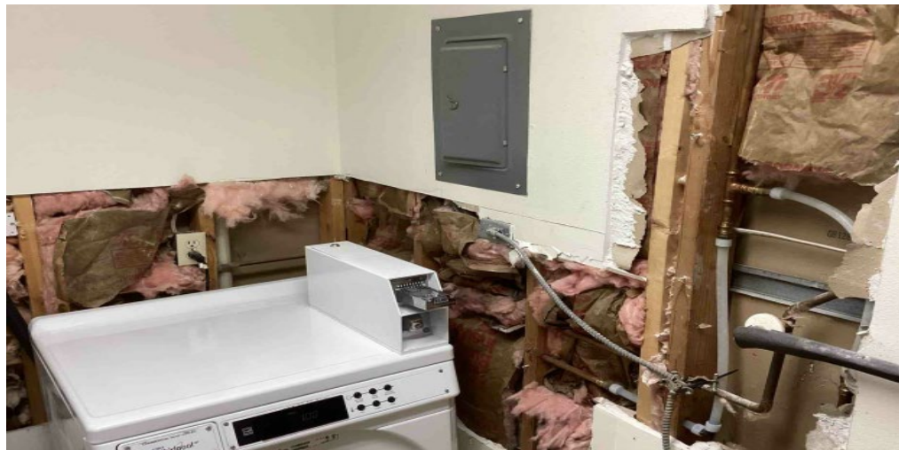
Figure 5: Photograph from RHS' records of an inspection performed at a sample project. The photograph shows the laundry area which has missing walls and a non-ground fault circuit interrupter outlet installed near a water source. As of December 31, 2025, these issues remained unresolved for 294 days after RHS notified the borrower.
