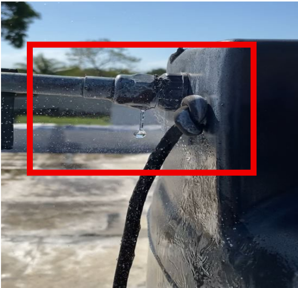
The picture above shows a water tank leaking.
