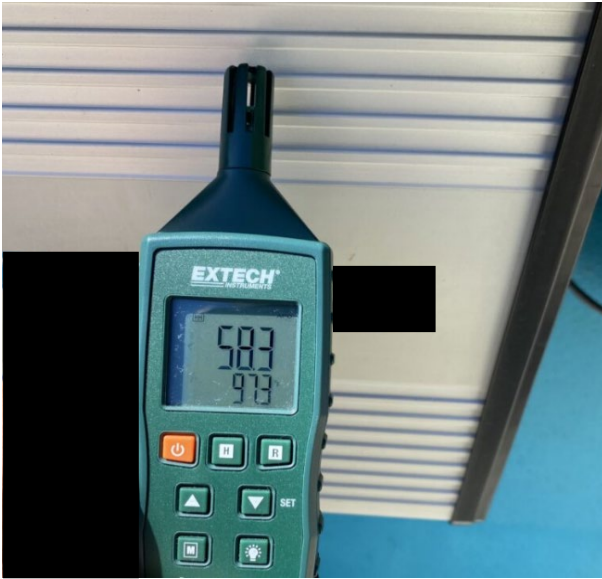
The picture above shows a battery directly exposed to temperatures of over 97 degrees Fahrenheit.
