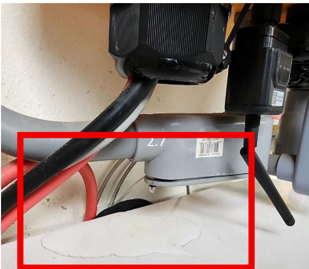
The picture above shows water leaking through the conduit and pooling on top of the battery. Specifically, water intrusion into electrical components could lead to electrical shorts and equipment malfunction.
