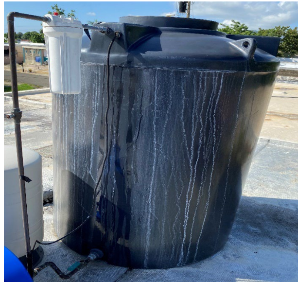
The picture above shows water stains on the tank due to the overflow.
