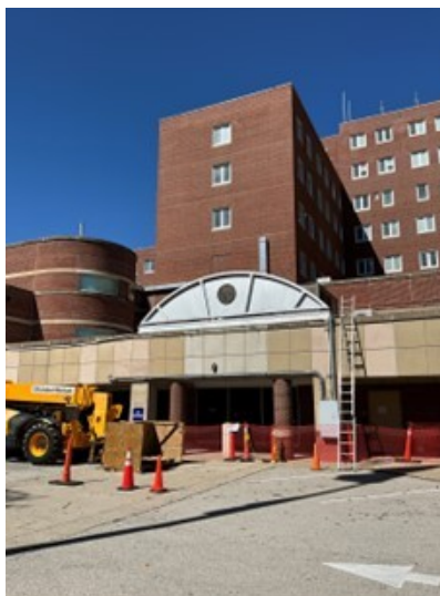
Figure C.4. Unattended ladder at clinic entrance.
