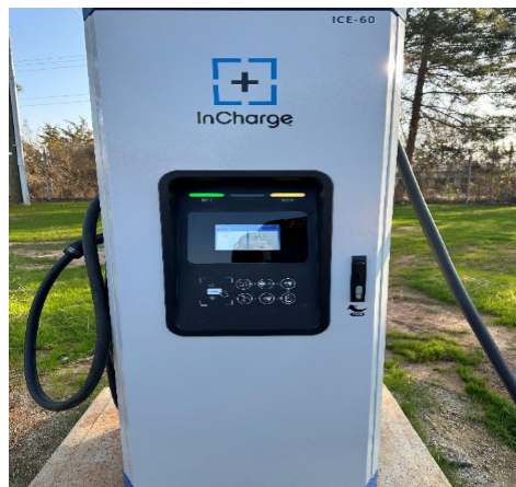
Front view of white electric bus charging station in South Carolina. (EPA OIG photo)
