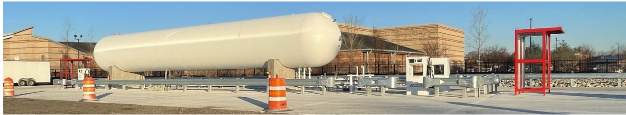
View of a white propane tank being installed in a parking lot for new school buses for Toledo Public Schools in Ohio. (EPA OIG photo)
