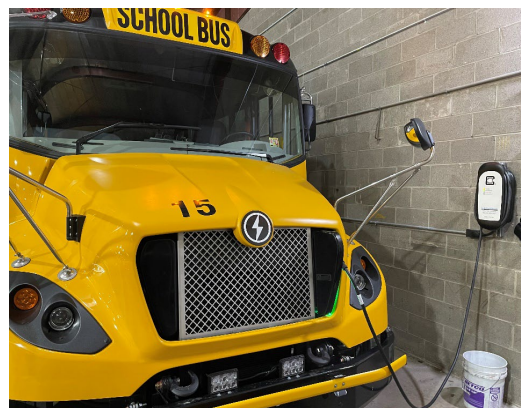
Electric bus temporary charging station. (EPA OIG photo)
