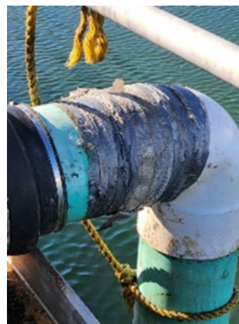
Example of poor maintenance of pipes using duct tape at the traditional side of the O.B. Curtis plant. (EPA OIG image).
