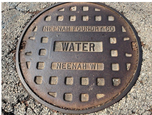
Source: EPA OIG image of a manhole cover in Illinois.
