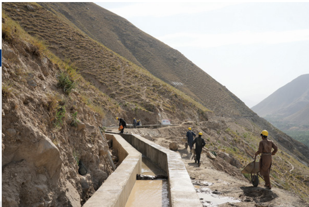
The Korkho ir Program anal under construction in Badakhshan Province. (WFP photo)
