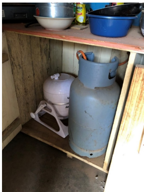
Figure 1: The deceased Volunteer's gas tank in its location in an improvised kitchen.
