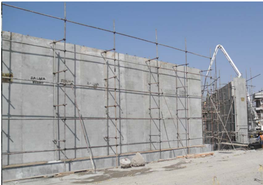
(U) Figure 1: Reinforced wall under construction at Embassy Kabul. (Photo taken by OIG, October 2017)
