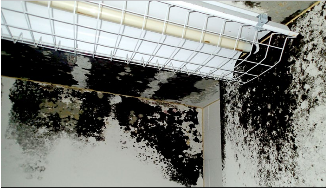
Figure 6. Unmitigated mold growth at Osan Air Base, Korea (not included in NOC). (Deficiency No. OSA-EN-140407-007) Source: Report No. DODIG-2015-013
