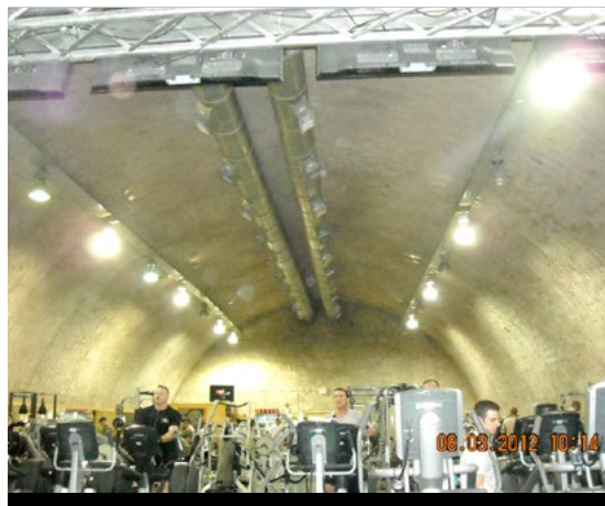
Figure 3. Unencapsulated flammable insulation at Bagram Air Field, Afghanistan. (Deficiency No. BAF-FP-120709-241) Source: Report No. DODIG-2013-099
