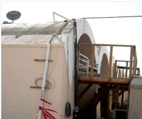
Figure 2. Live wires directly on roof at Kandahar Air Field, Afghanistan. (Deficiency No. KAF-EL-120426-084) Source: Report No. DODIG-2013-099
