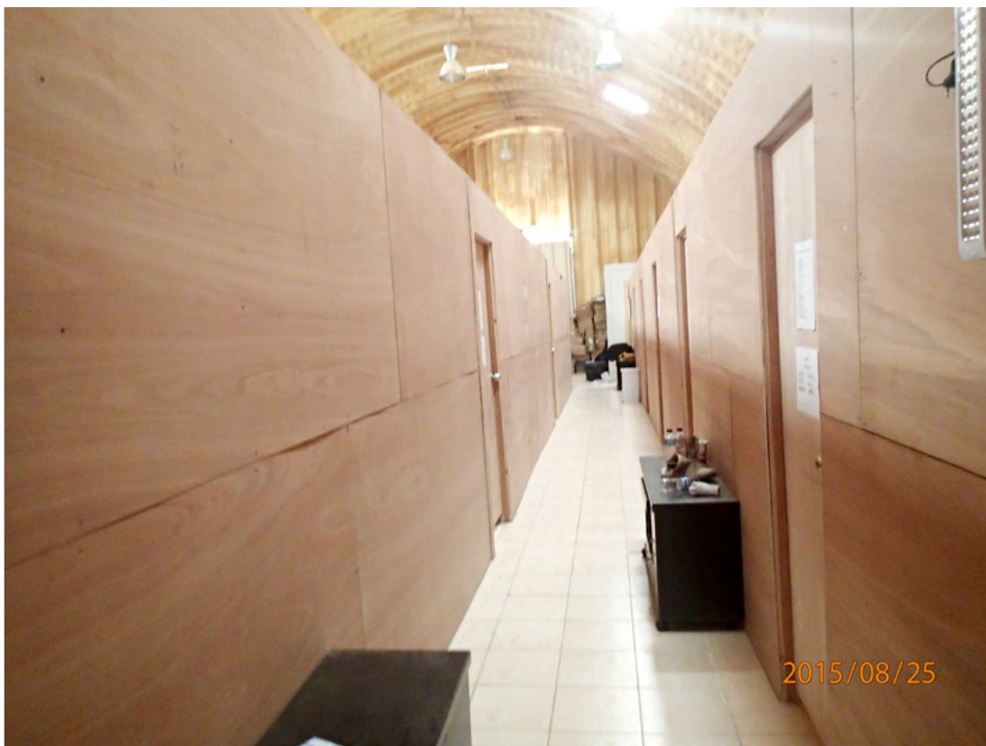
Figure 8. Building with no sprinklers that also lacked required fire-rated construction at KASOTC, Jordan. (Deficiency No. KAS-FP-150828-134) Source: Report No. DODIG-2016-106
