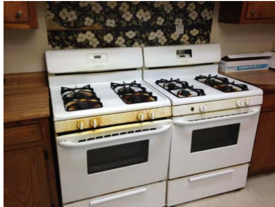
Damaged kitchen stoves (broken oven controls, broken oven door, and missing stove knob)
